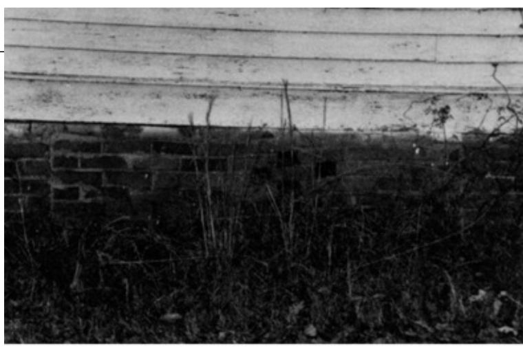
Wavy lines along rows of bricks indicate the foundation has sunk. Also, the clapboard siding is rotting along the foundation.
