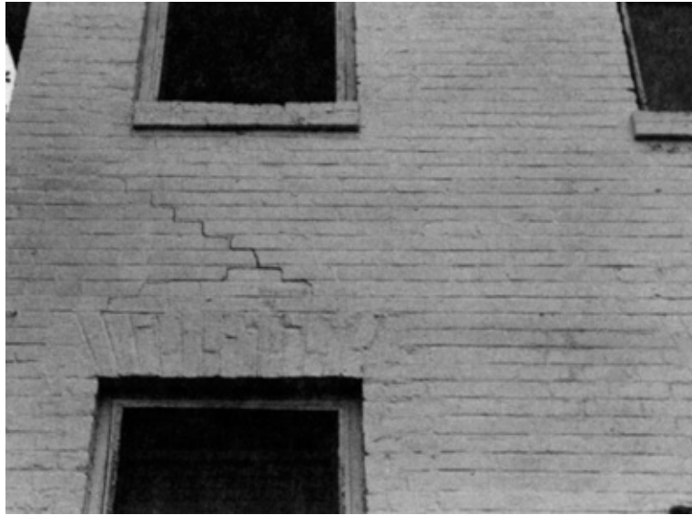
The pattern of cracks in the bricks shows this corner of the house has sunk.
